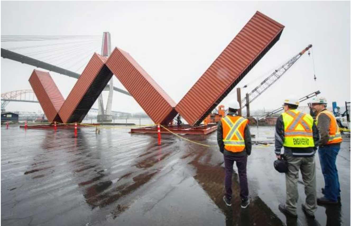
Workers finish placing the WOW Westminister art installation on the New Westminister waterfront Monday. WOW New Westminister, by José Resende, is one of the Vancouver Biennale outdoor artworks and consists of four 40-foot high shipping containers cantilevered into the shape of a 'W.'
