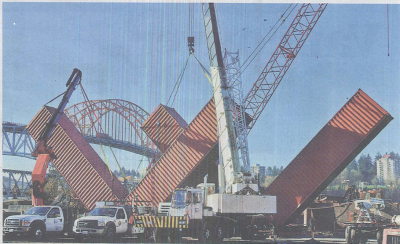
PIER PARK VANCOUVER BIENNALE SETS UP NEW ART PIECES Crews prepare shipping containers for a piece of public art called Wow Westminster. The art will be installed at Pier Park in New Westminster on Monday as part of the Vancouver Biennale. RIC LAM/ROAMING THE PLANET
